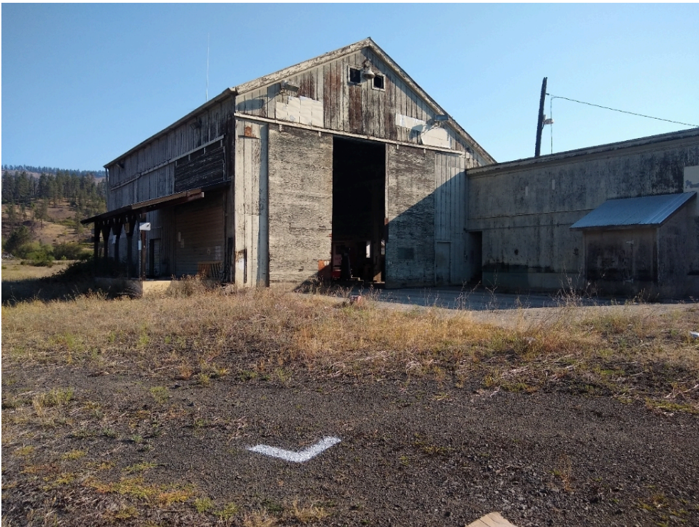
Photo Location: West of tracks, southwest corner of building. Looking Northeast Photo Description: GCP 4
